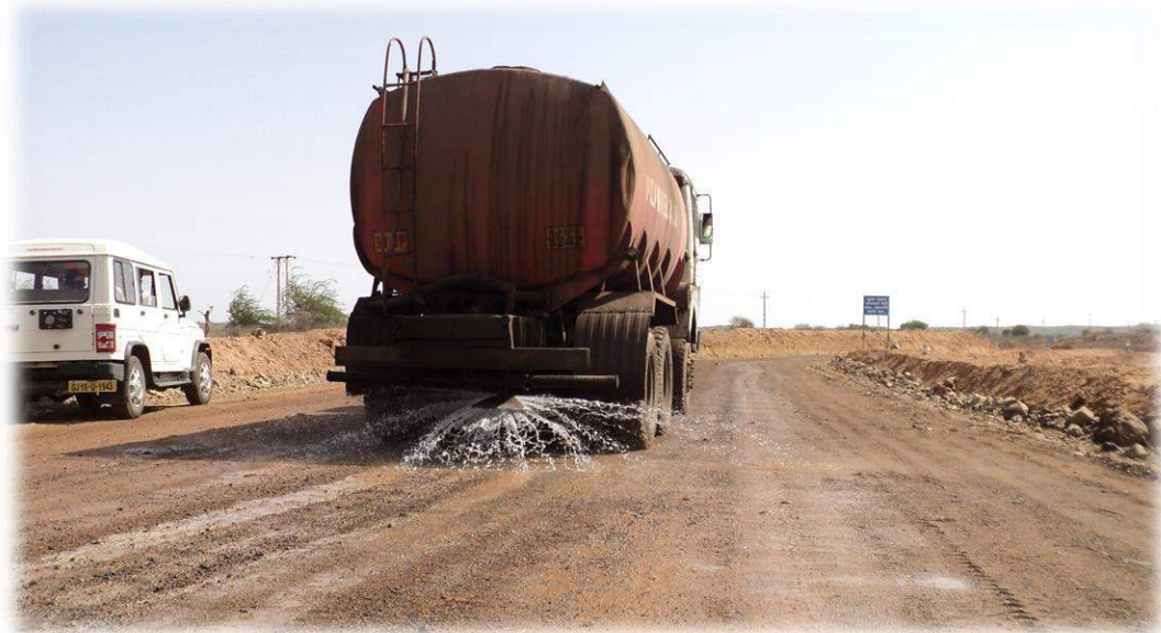
Water sprinkling system provided to check dust emissions at haulroad.
